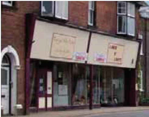
Poor quality shop fronts along West Street
