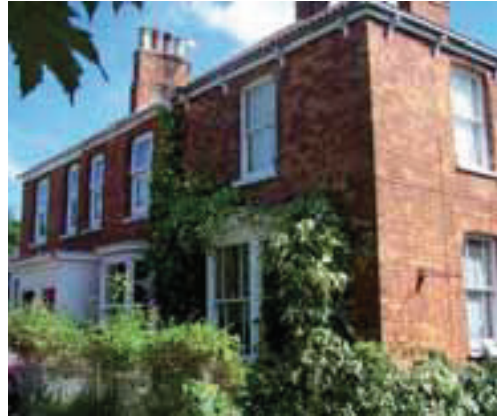
Quarry Road – contrast in quality of detailing between original and replacement windows
