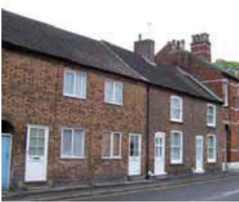
Gospeigate – erosion of traditional detailing with replacement windows and roof covering and loss of chimneystack
